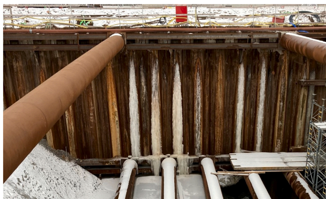
Fig. 18. Leakage from the joints of SPW (Bozkurt, Sinem. West Link project, Gothenburg. 16 Feb. 2021. Author's personal collection).
