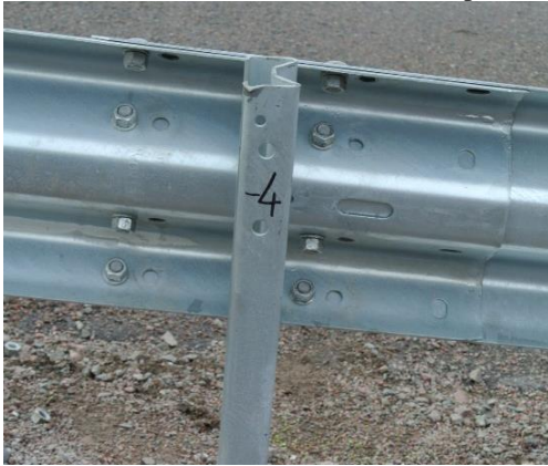
Figure 10. New holes made in one of the overlap joints to compensate for the gradual stretching of the guardrail.
