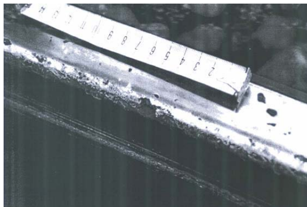
Figure 4: Spalling in rails [Courtesy - Mats Rhen and Dan Larsson, LTU]
