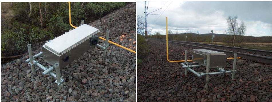
Figure 14. T/BOGI installation at Kiruna during field test.
