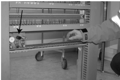
Figure 11. The placement of the RC circuit in the rack (the middle RC circuit in the square indicated by the arrow) and the wire from RC circuits that have the same size both on the negative bound and on the voltage side. The area of the solid wire is 0.75\ \text{mm}^2 .
