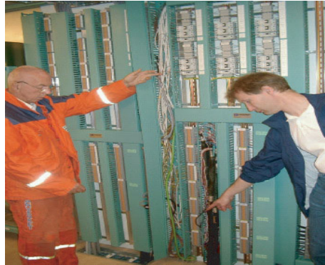
Figure 3: Incoming cables in a technical building where the overvoltage protection filter is placed over 1 metre from the wall that is the barrier. The unfiltered cable is mixed with filtered cables before it reaches the overvoltage filter.
