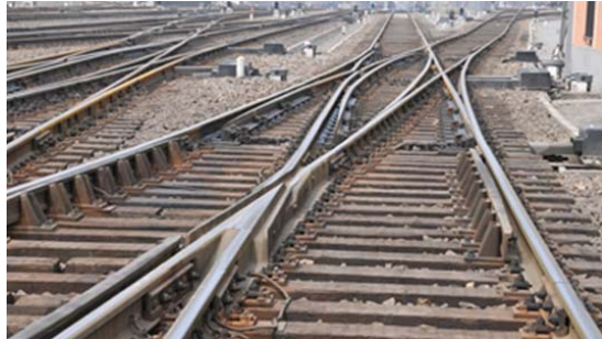
Figure 5. A kind of Switches and Crossings
