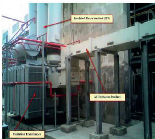
Figure 5: Actual busduct location at site
