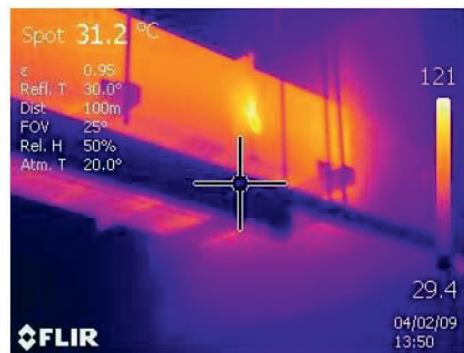
Figure 8: Hot spot temperature around the jumper cable connection
