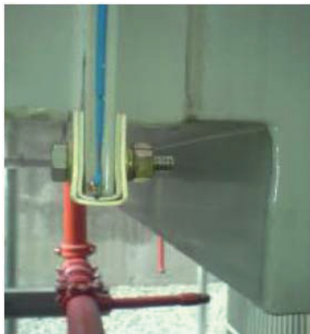
Figure 9: Copper plates on the flange connection
