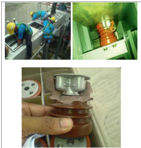
Figure 7: Damaged post insulators inside the busduct
