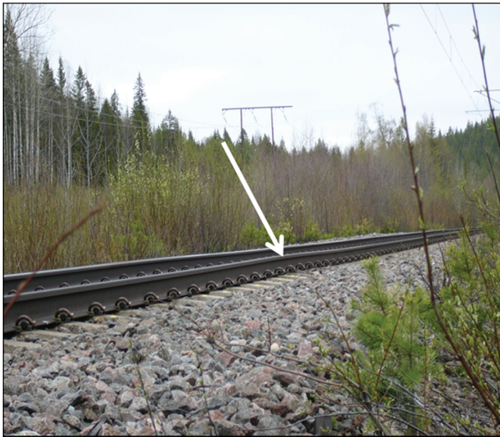
Figure 10: The effect of culvert on the track geometry
