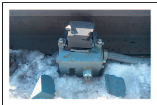
Figure 9. Failed sensor belonging to the wheel profile monitoring system (photo by Dan Larsson).
