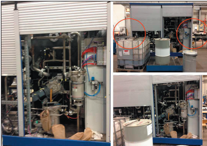
Figure 63. Machine for degreaser bath.
