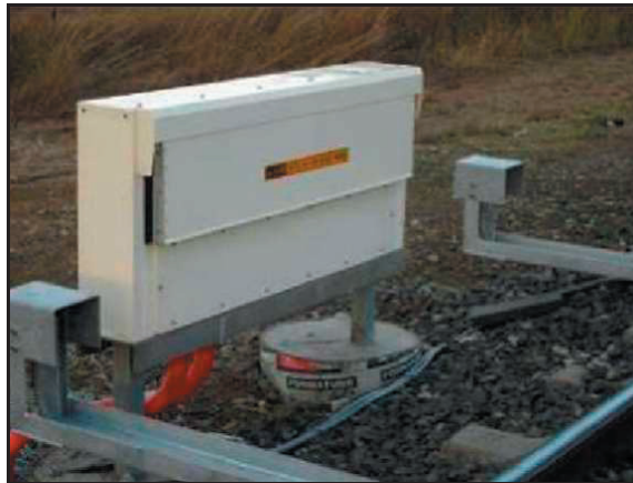
Figure 17. Microphone station. (Vipac Engineers) [26].
