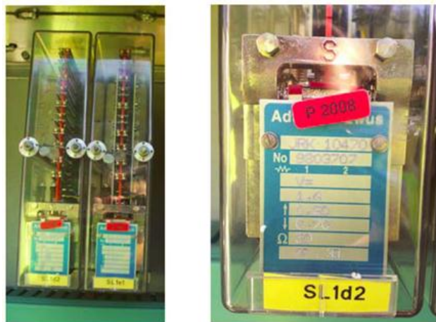
Figure 1. Detail of the most used relay in Sweden, model JRK 10470.
