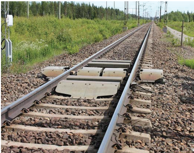
Figure 4: Wheel profile measurement unit installed in the southern part of the Iron Ore Line.
