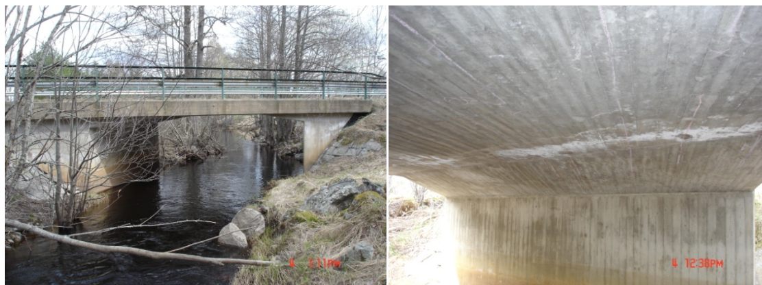
Figure 5.4.13 Concrete bridge 19-117-1 [Lind & Wikslund, 2010] (Left: a view from side; Right: Lime precipitations underside the bridge slab).
