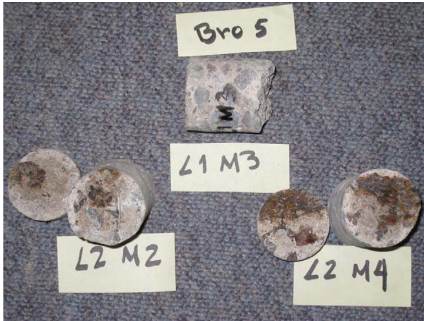
Figure 5.3.7 Corrosion on the steel bars in cores L2M2 and L2M4 drilled from Bridge 5.
