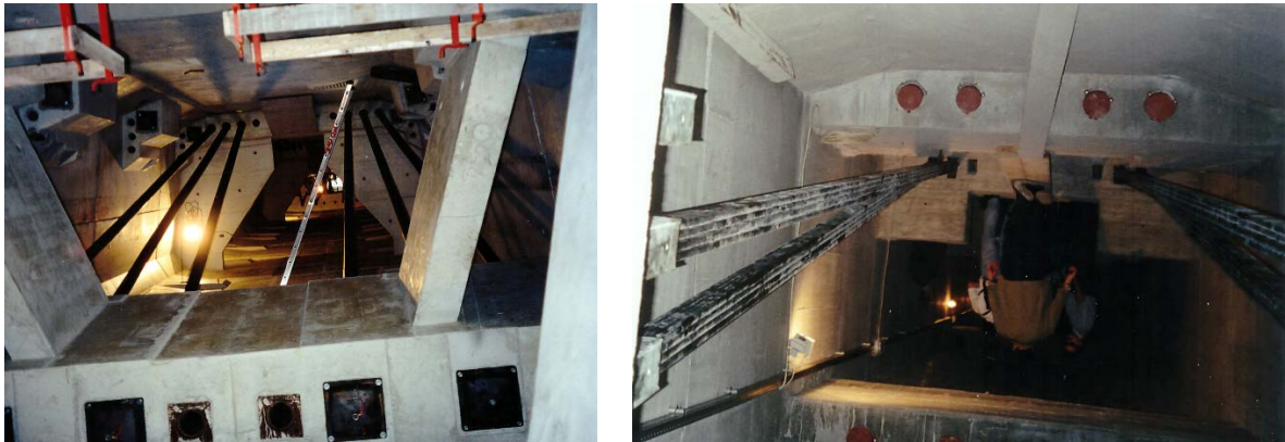
Figure 7.4 External post-tensioning applied to concrete box-girder bridges Photos from a French bridge on high speed line to Marseilles left and a Hungarian bridge on the new freight line through Slovenia to the Mediterranean (Photos by B. Paulsson)
