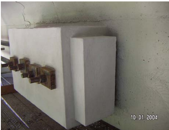
Anchor block for two cables. Shear face is prestressed by 4 transverse bars
