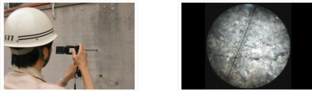
Figure B.10 Use of endoscope identifying a crack in concrete, from ( http:// www.nishimatsu.co.jp )
