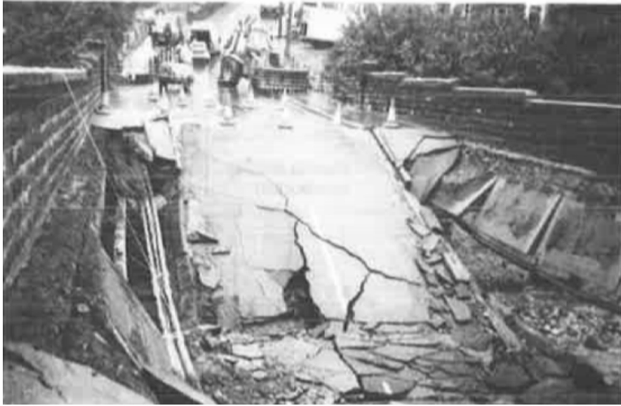
Figure 3.6. Collapse of bridge in Wales 1985. Woodward (1989).
