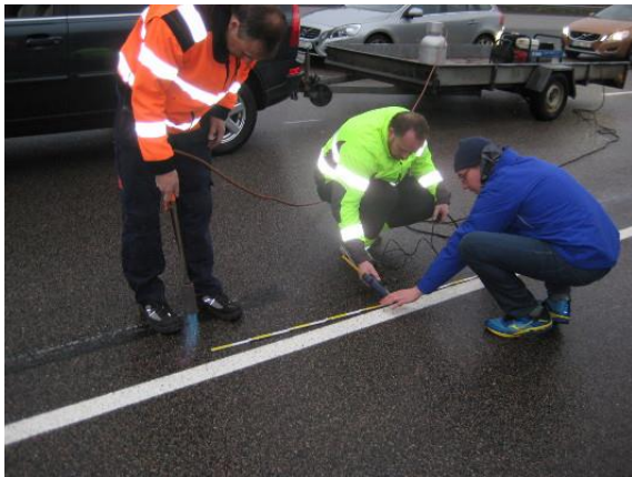
Figure 19 Gluing the magnets to the pavement for the high speed test, the torch was used for drying the pavement.
