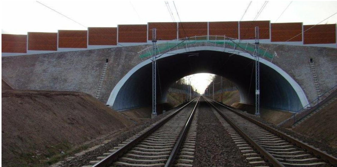
Figure 2.2 By completing the steel structure with well-designed details, nice looking bridges can be achieved. This bridge is one of the largest SSCB in Europe having a 20 m span.
