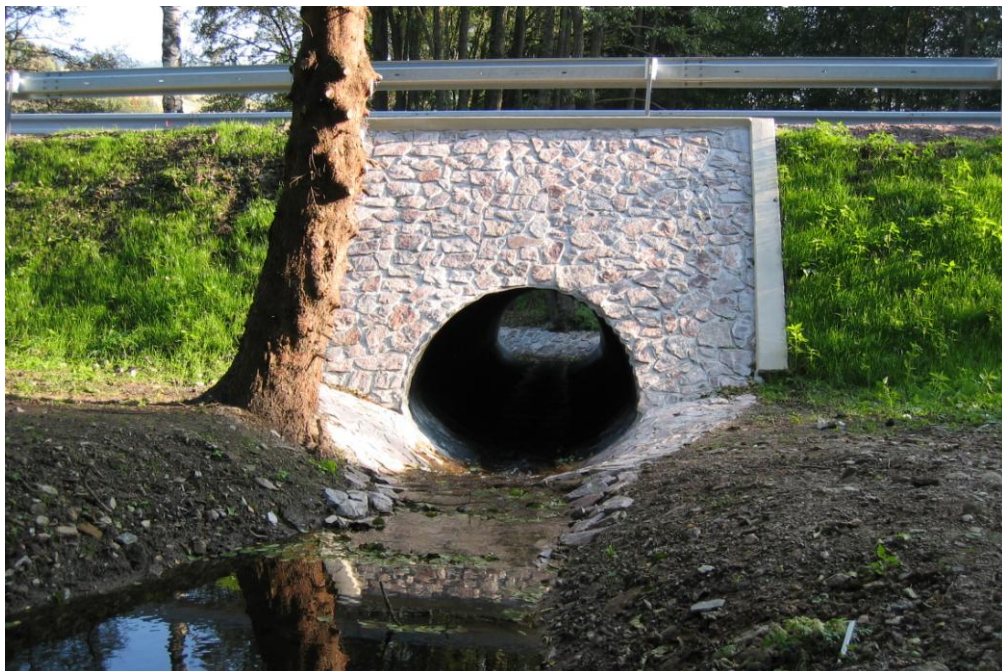
Figure 2.3 A nicely worked out glacis covering the slopes of a pipe-arch bridge.-
