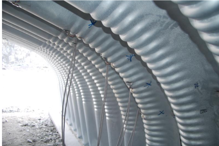
Figure B1.1 Photo showing so called cross corrugation (from the Järpås full scale tests).
