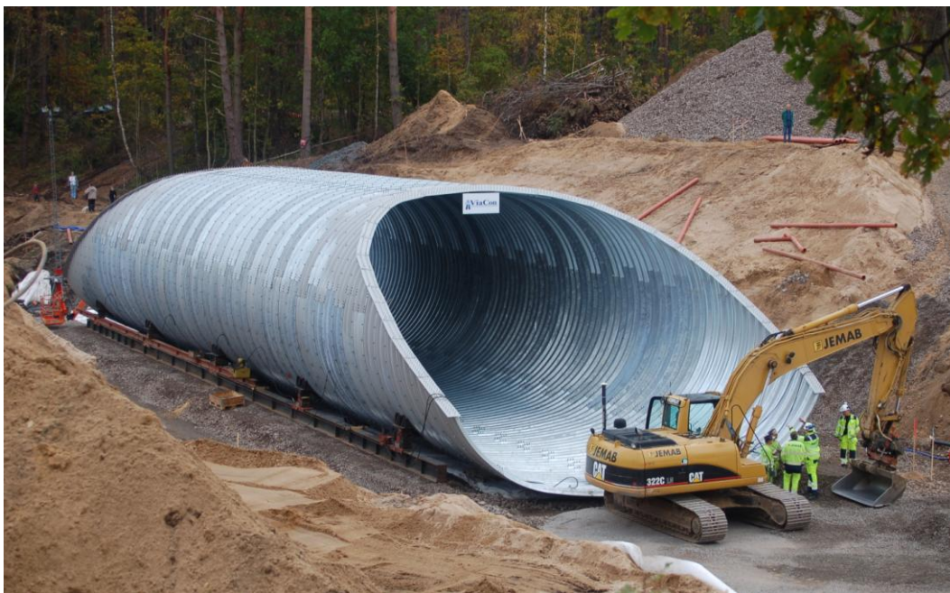
Figure 2.1 The finalized erection of the steel part of a SuperCor pipe-arch bridge, see Figure 1.3 B, just before starting the backfilling process.
